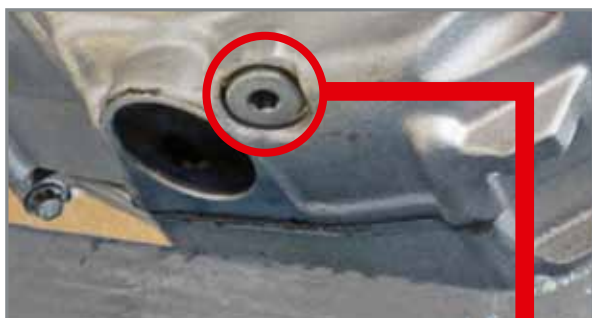
Location of pressure control valve.
